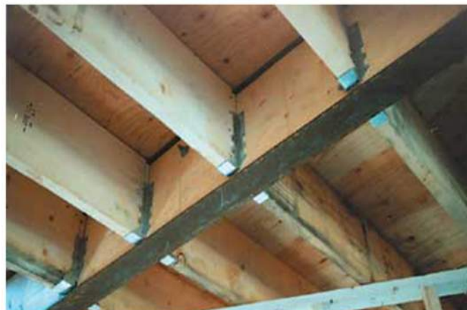
Above: An example of substring construction, where I-beams are holding wooden ceiling.
