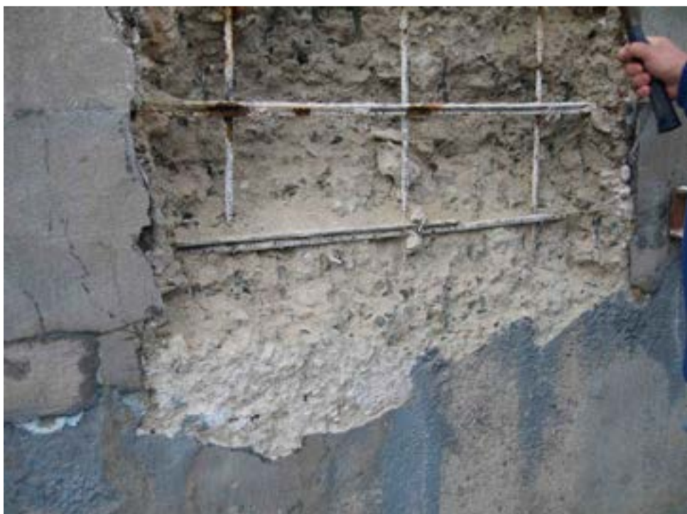
Concrete damaged surface exposing iron rebar
