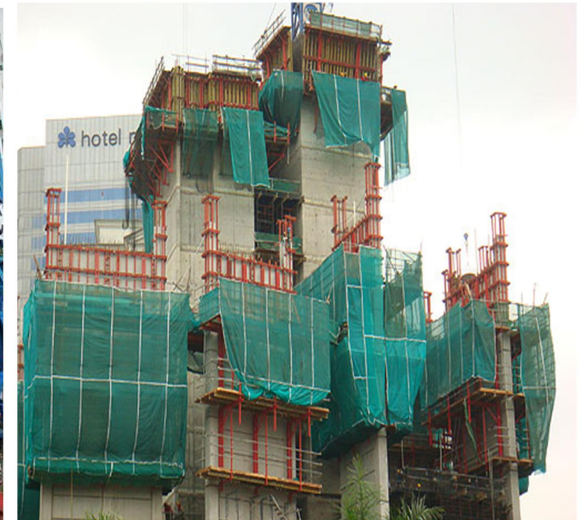
The casting height is control by the precast arrangement ranging from 1 precast to a maximum of 3 precast at one time. The average height of a precast panel is 1.137m.
