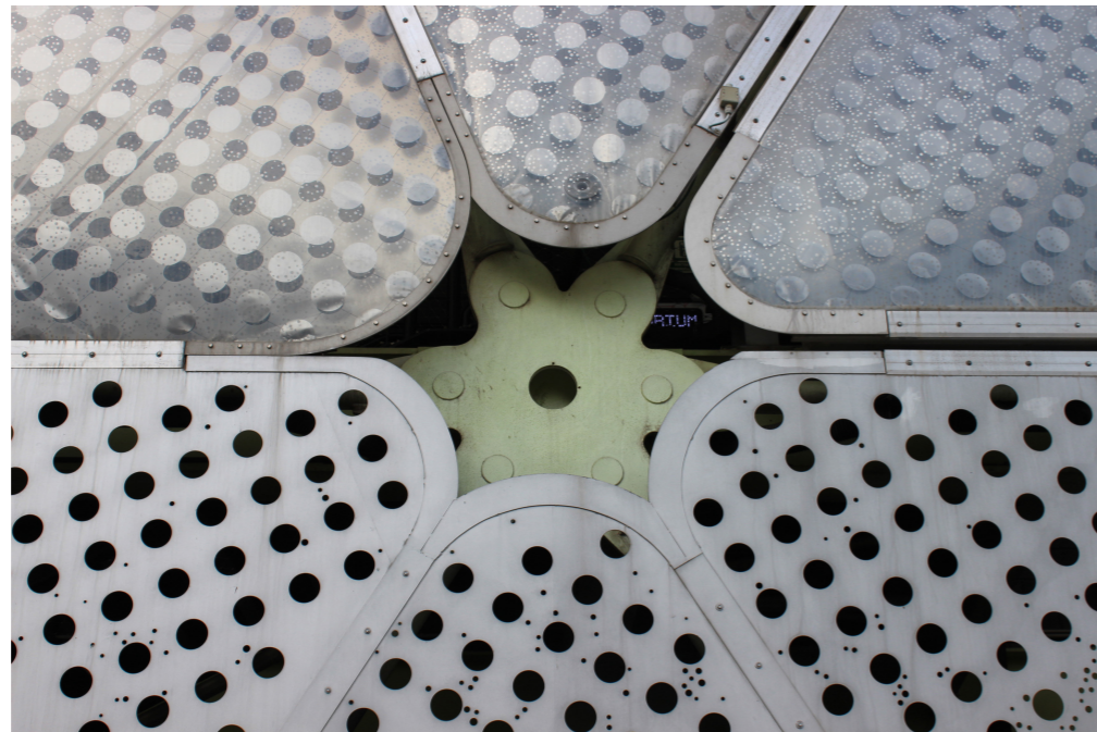
Image 2 Close-up of the ETFE panels connection point, and struc- tural pinned-connection behind the façade
